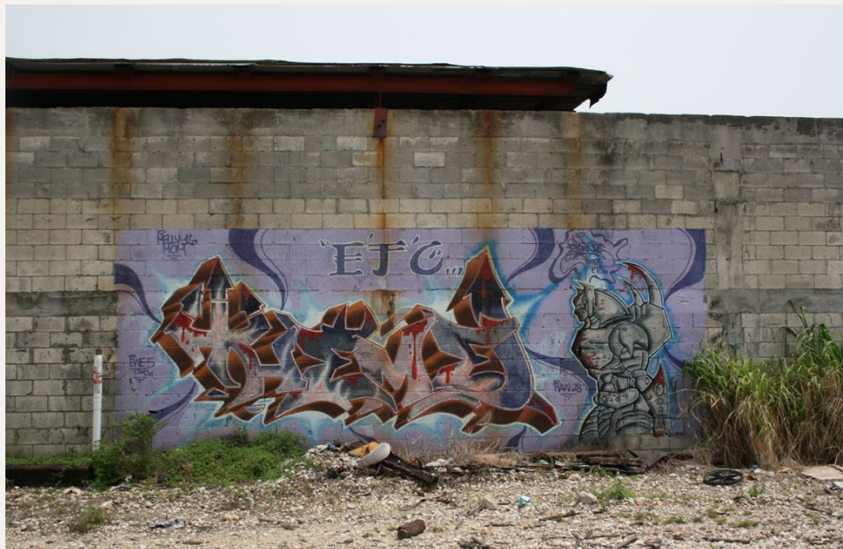
Figure 30: Graffiti 'art' on masonry wall.
